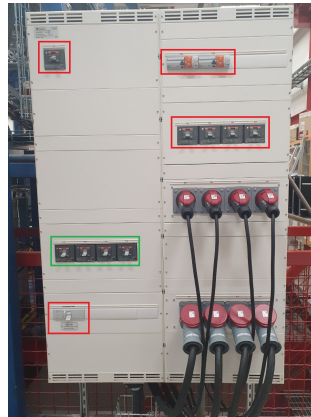
Figure 4: Fuse box for the Keysight hardware.
